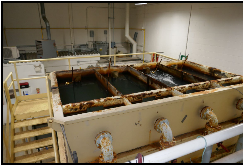
Interior of the Treatment Plant
