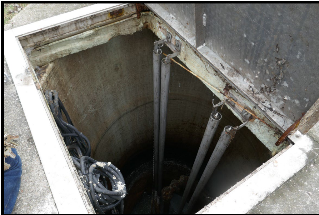
West Lift Station
