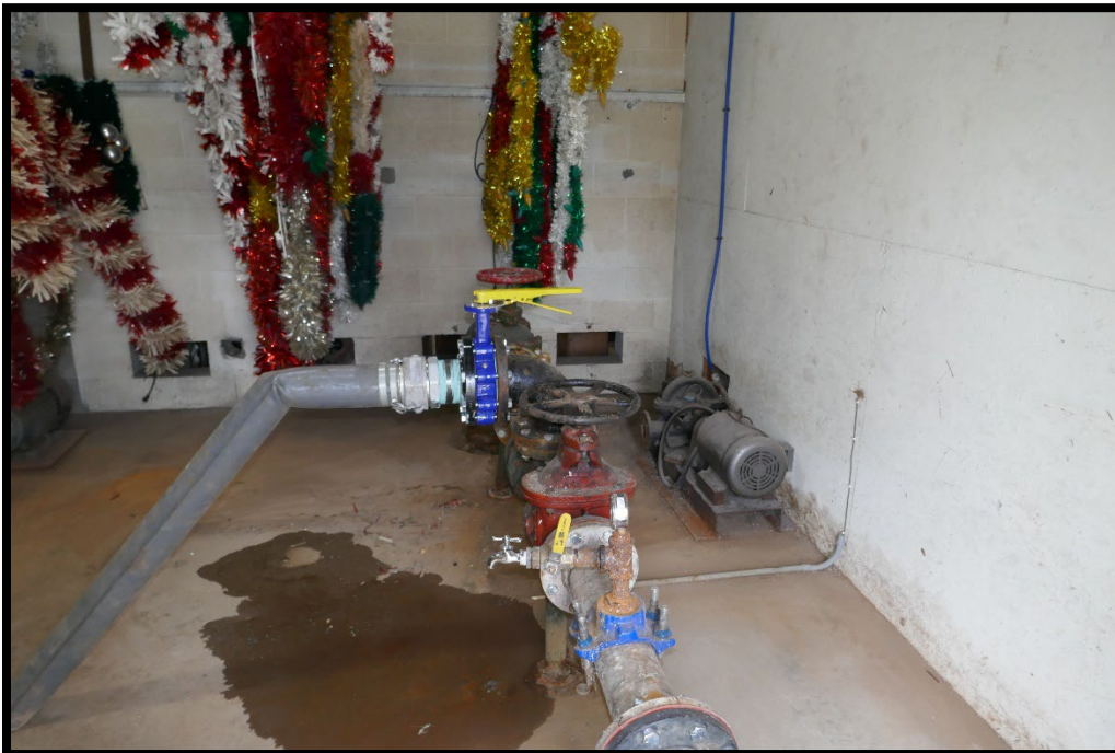
Main Well – Located in City Maintenance Building
