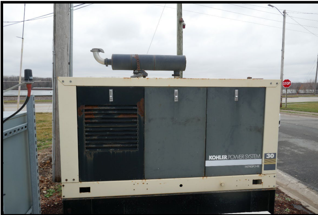
East Lift Station
